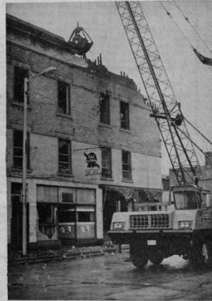
The Janesville Construction Co. was called to the burned-out structure late Monday afternoon and began demolition work. The back of the building already had caved in, and, because he feared the front may do the same because of the large amounts of water poured on the building, Edgerton Fire Chief Norman Yeske ordered everyone to stay clear. A few items were recovered at the businesses.
