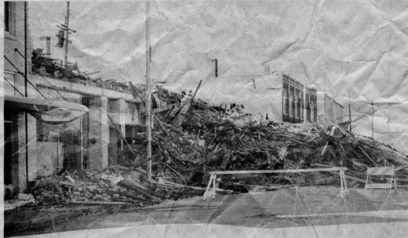
Tuesday morning, the former Schmeling building in downtown Edgerton still remained in a heap in the middle of Henry Street. Owner Miles Durfee, Janesville, was given 48 hours to remove the rubble upon condemnation.
